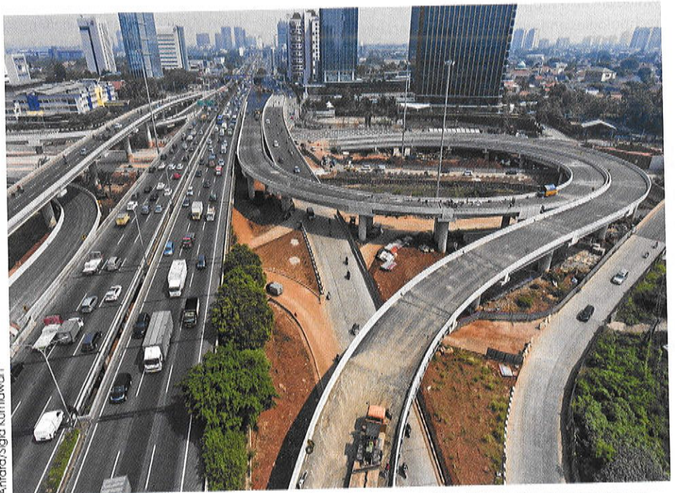
Final stage: The construction of the Antasari interchange, part of the Depok-Antasari (Desari) toll road linking South Jakarta and West Depok, is currently in its final stage. Building toll roads is part of the government's infrastructure development program.
